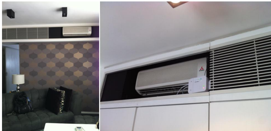
Figure 1. COOLNOMIX Installation in Apartment 18B
